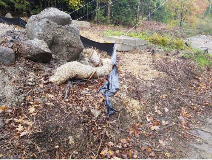
Fig 13: Silt fence near Str. 29 need repair. Viewing north. (10-08-019).
