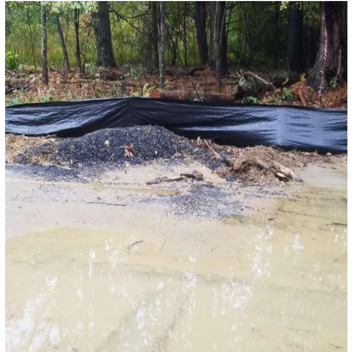
Fig 4: Cold patch needs to be removed from the site. Viewing south. (10-08-19).
