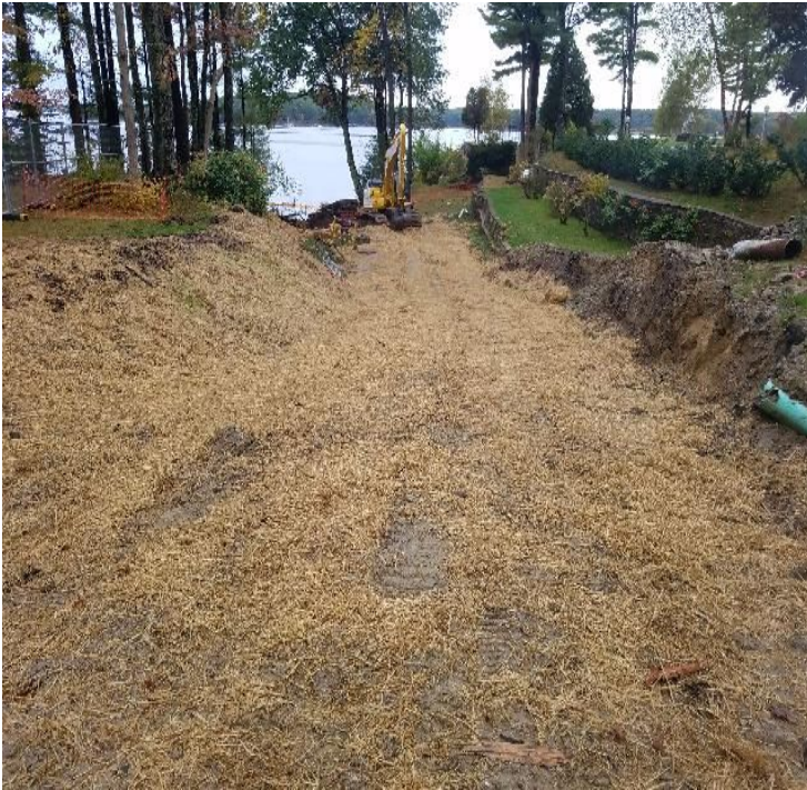
Fig 5: Exposed soil covered on the slope at the Beswick property. Viewing west. (10-08-19).
